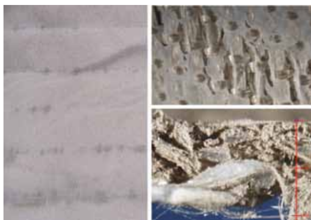
Figure 6. Membrane laminated onto woven glass after 29 months' operation in a clinker mill filter. (Left: clean gas side, right: cracks in the membrane and cross-section.) Surface filtration is achieved as long as the integrity of the surface is maintained.
